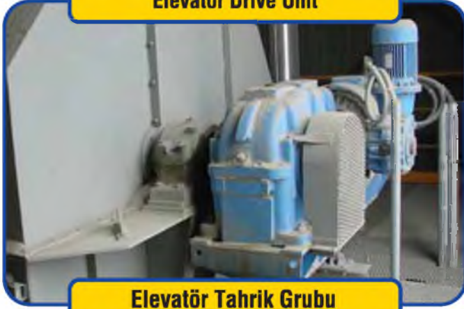
Elevator Drive Unit
